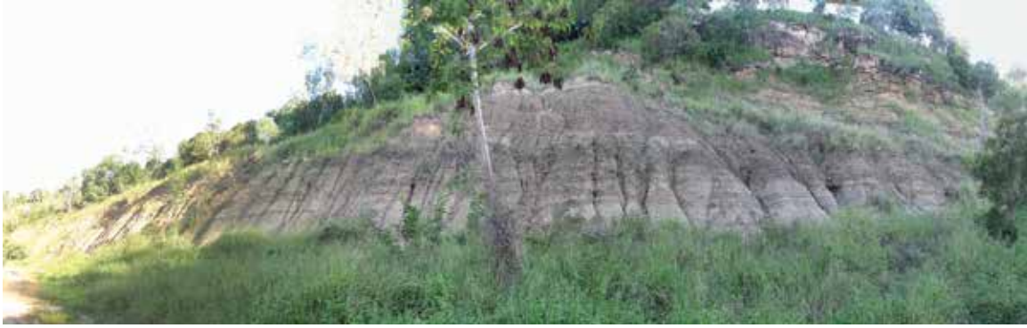
Pt. 3. Panorama of cutting about 1 km east of Lowood in friable sedimentary rocks (Gatton Sandstone at the foot). Total height about 30 m. This cutting was set back about 10 m from the rails, so that minor landslides would not block the line.
